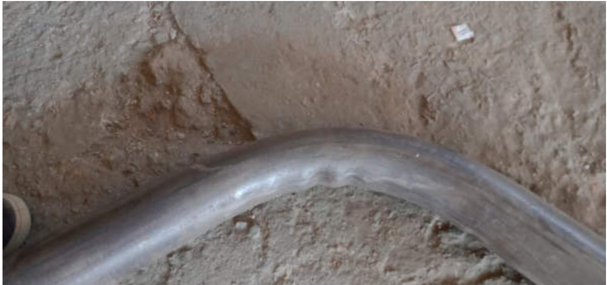
Fig:2.10 80 mm Pipe With Wrinkles
