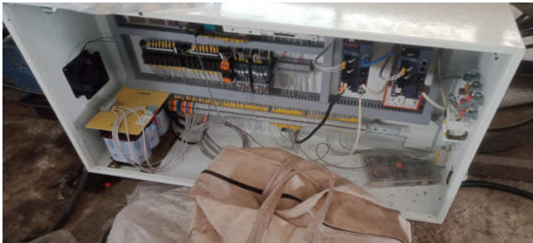
Fig 4.16 PLC Panel Connection
