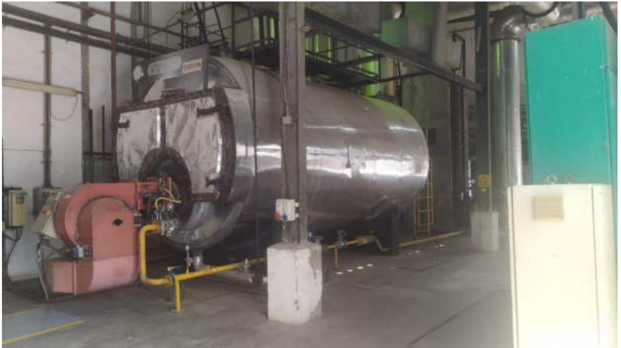
Figure 3.10 Line 1&2 Boiler Room
