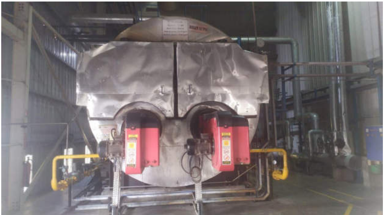
Figure 3.11 Line 3 Boiler Room
