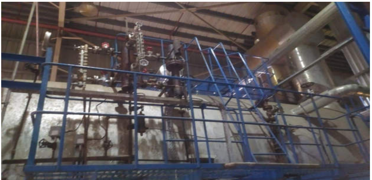
Figure 3.3 Water Level Indicator
