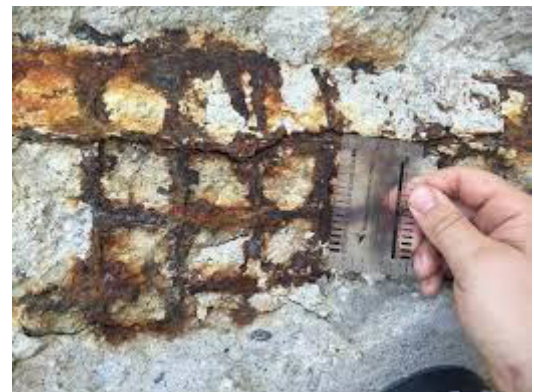
Figure 40 Chloride induced corrosion
