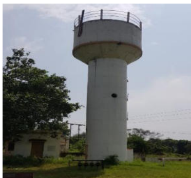
Figure 14 Over head tank
