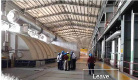
CGPL 800 MW TURBINE HALL
