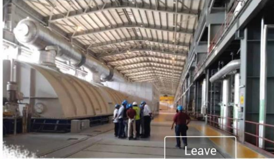
CGPL 800 MW TURBINE HALL
