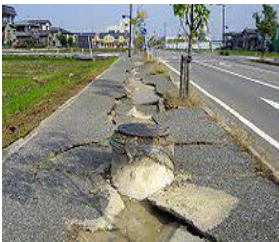
Figure 35 Soil liquefaction on road
