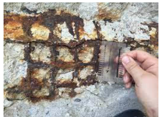
Figure 40 Chloride induced corrosion
